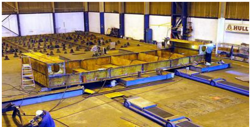
Northrop Grumman Newport News employees will build the USS Monitor replica in 22 steel sections inside the shipyard's steel production facility. Pictured is the first section, called the keel unit, which weighs approximately 18 tons and is about the size of a rail car.
