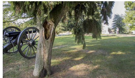
This Fraser Fir is one of the trees that will be removed from the Soldiers' National Cemetery due to safety concerns. It has a hollow trunk and there is a vertical crack that is further weakening the trunk.
