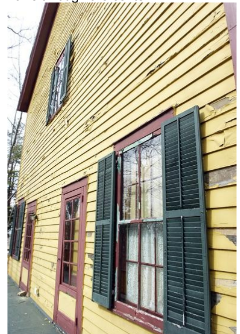
The elements have chipped away at the paint on the south side of the Ulysses S. Grant Cottage. (ERICA MILLER/The Saratogian)
