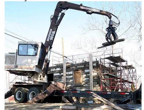
A huge mechanical claw carefully removes timbers from the William Patterson House along Taneytown Road on Thursday morning. The two-room log structure, built in the 1820s, is the oldest house located within the boundaries of the Gettysburg National Military Park. Park employees will replace deteriorating components and reassemble the building to its 1863 appearance. (NPS Photo)
