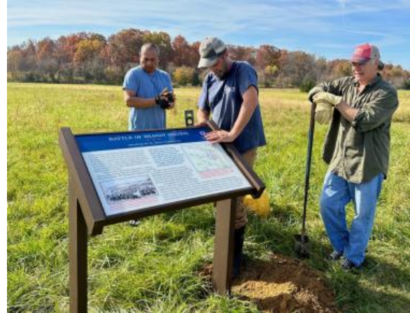
New sign installations at Brandy Station Battlefield in Culpeper, Va. American Battlefield Trust
