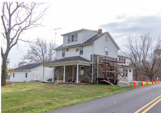
Selective demolition of modern additions at historic Warfield house to begin December 2.
