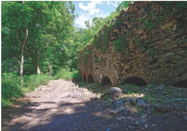
Union troops hid from hostile gunfire in these Boteler's Cement Mill kilns located along the Potomac River. Friendly Union artillery fire killed a number of them. (Photo by Melissa A. Winn)
